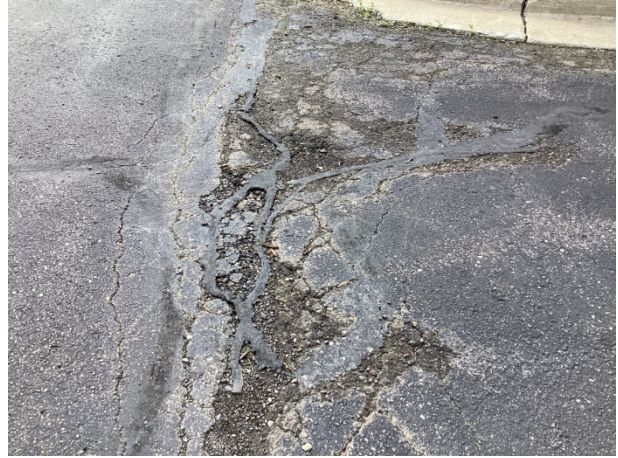
Pavement deterioration and failed repairs along Bent Trail Drive
