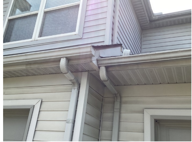
Aluminum gutters and downspouts
