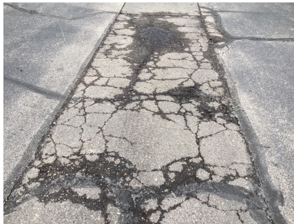
Alligator cracks along previously patched section along Bent Trail Drive
