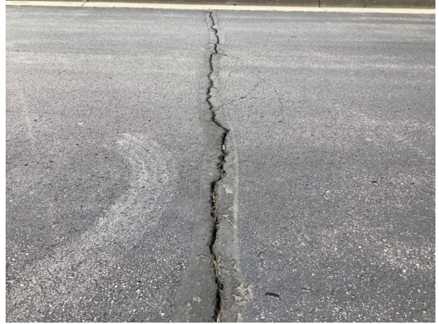
Pavement cracks along Bent Trail Drive
