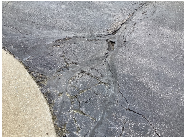
Alligator cracks and pavement deterioration along Bent Trail Drive
