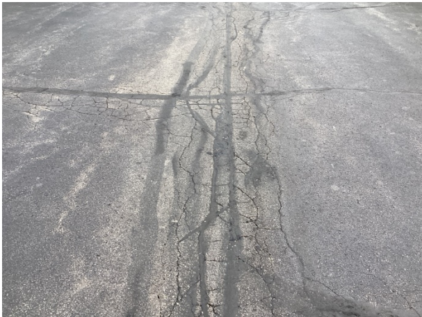
Previous repairs and alligator cracks along Meadow Grove Trail
