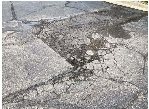
Alligator cracks along Meadow Grove Trail
