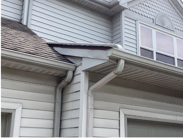
Aluminum gutters and downspouts
