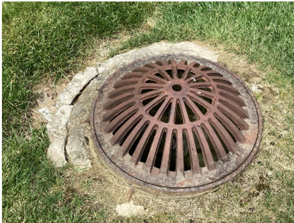
Catch basin along landscape- note collar damage
