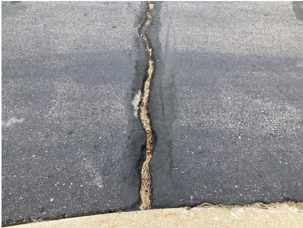
Pavement cracks along Meadow Grove Trail
