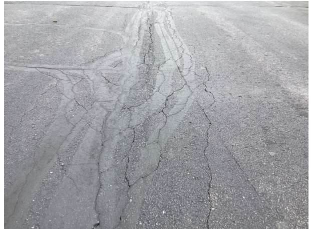
Alligator cracks along Meadow Grove Trail
