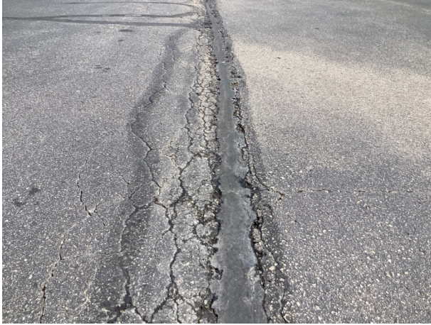
Alligator cracks along failed repairs along Bent Trail Drive
