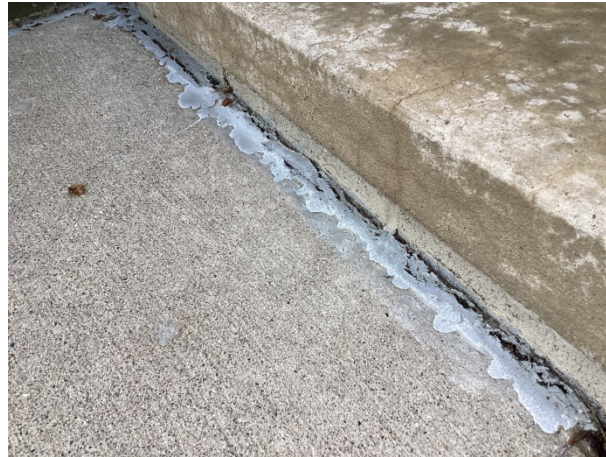
Sealant deterioration between sidewalk and stoop
