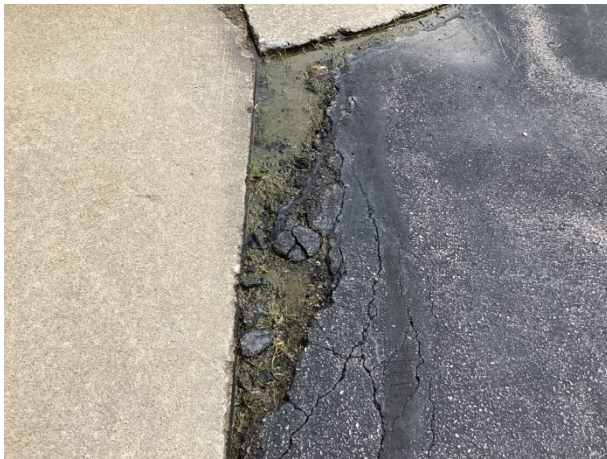
Edge deterioration and pooling of water at Bent Trail Drive
