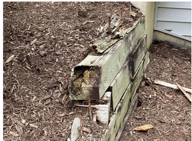
Wall wood rot
