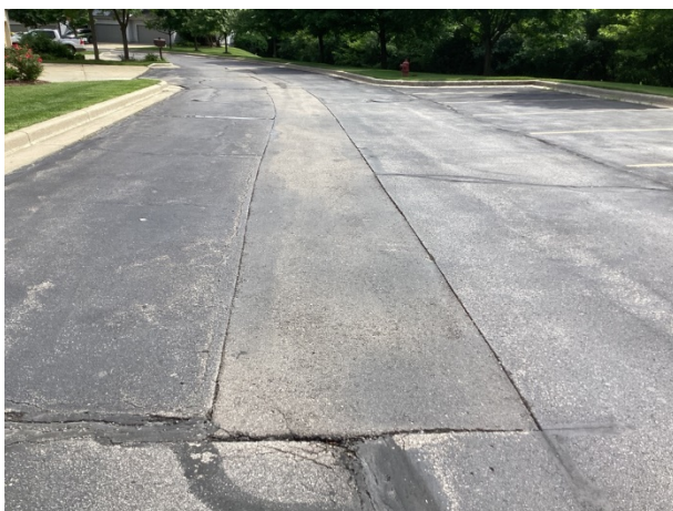
Previously patched section
