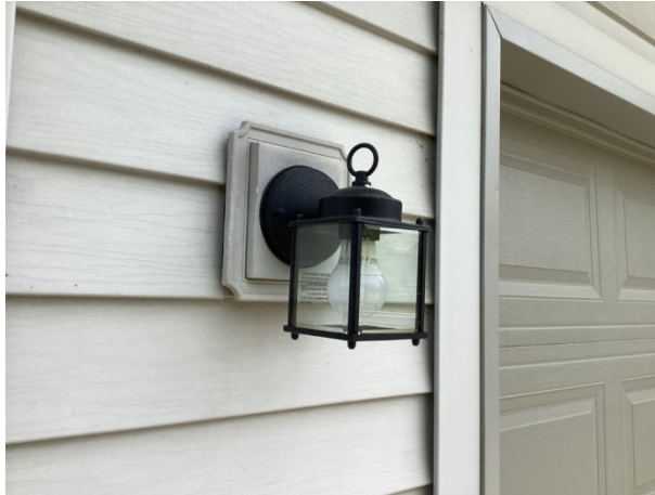
Exterior light fixture
