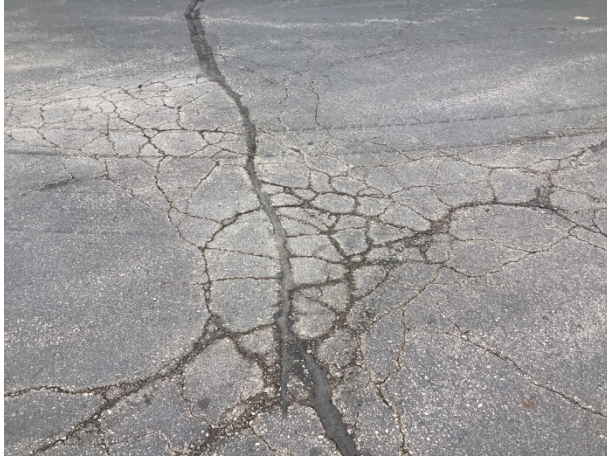
Alligator cracks along Meadow Grove Trail
