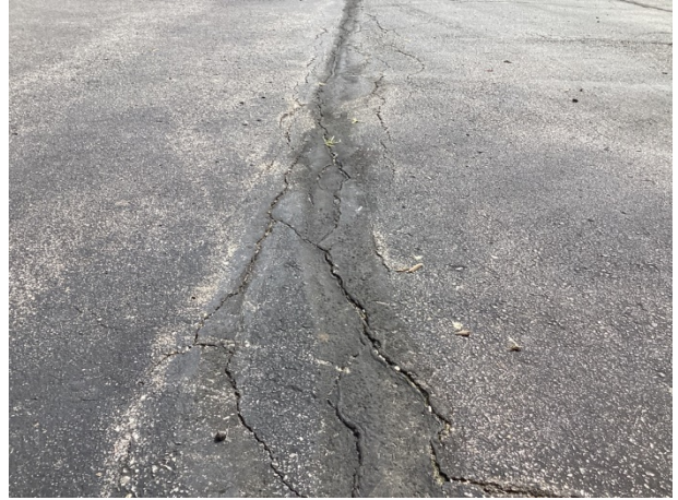
Pavement cracks along Bent Trail Drive
