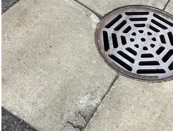
Catch basin collar damage
