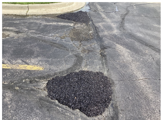
Pavement cracks and previous repairs
